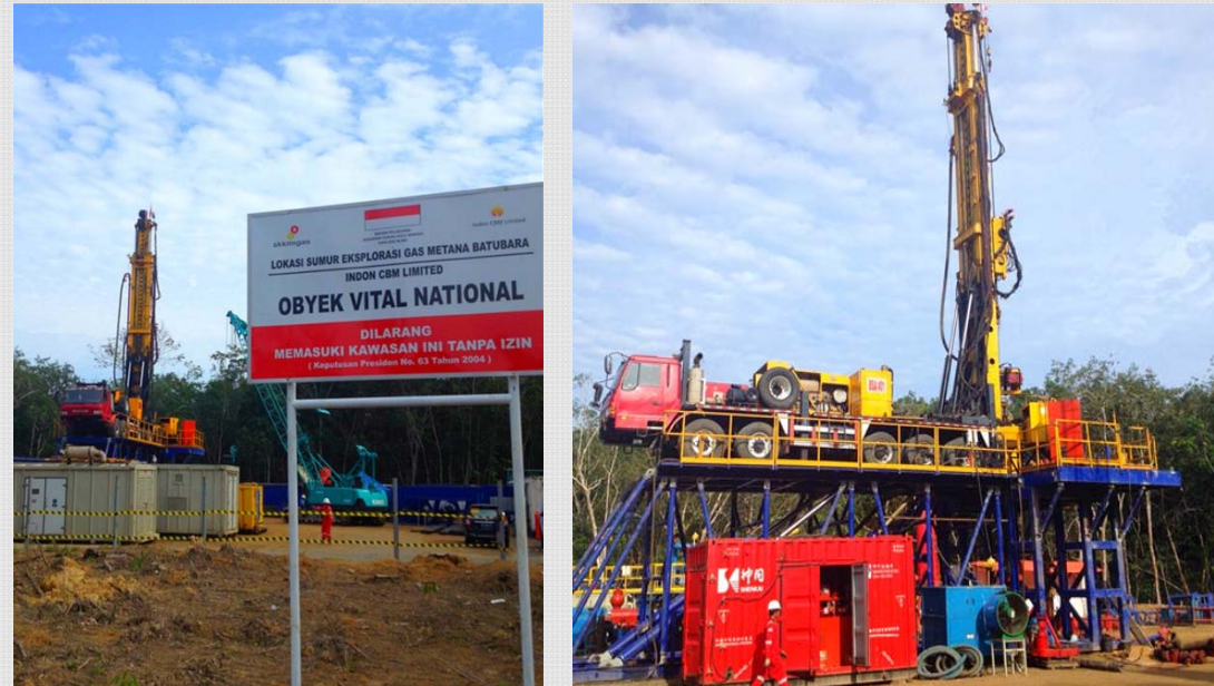
Well Site at RE-CBM-01CE
