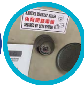
CCTV cameras in all buses
