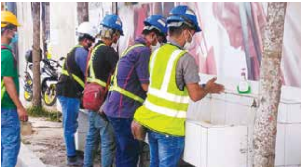
Hand-washing facility equipped with soap and clean running water for workers
