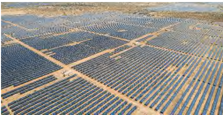
Bhadla Solar Park India
