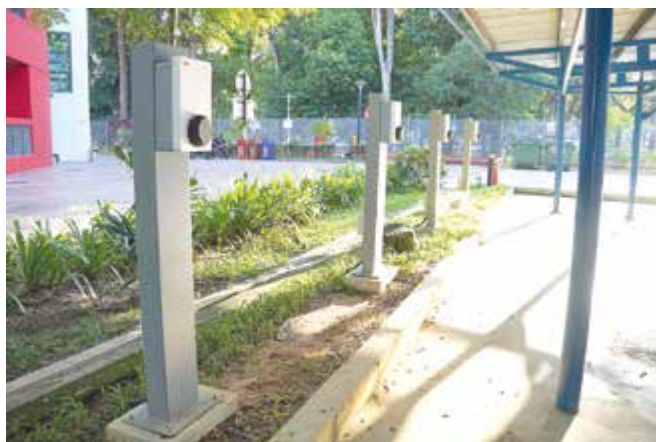
EV charging station to encourage green vehicle adoption
