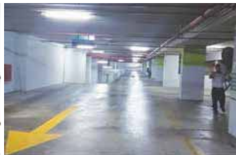
Figure 28: Installed energy efficient LED lighting
