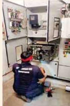
Figure 18: Major service and maintenance work of high tension and low voltage electrical panel at the building
