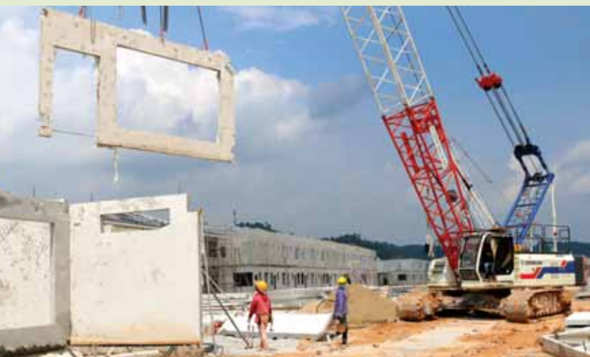
Implementation of IBS system in development of landed residential homes in Hillpark @ Shah Alam North
