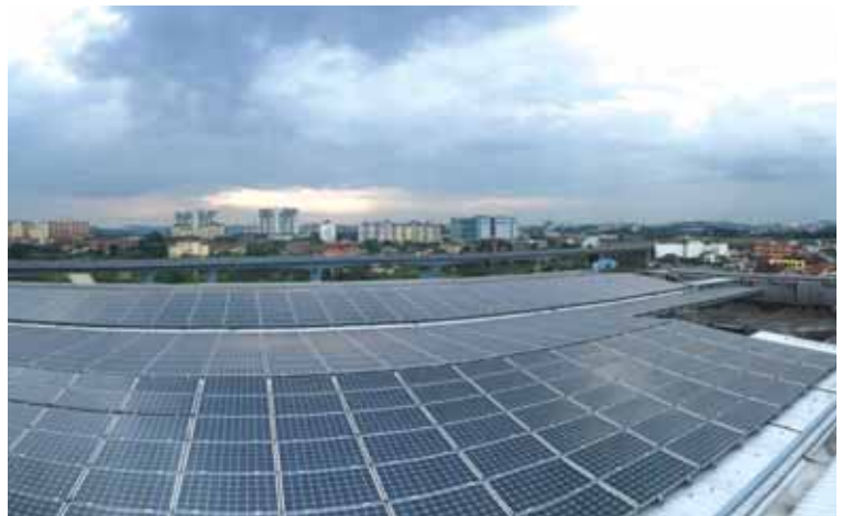
The solar photovoltaic panels installed on the rooftop of Plaza Metro Kajang is estimated to reduce electricity consumption by about 10% annually
