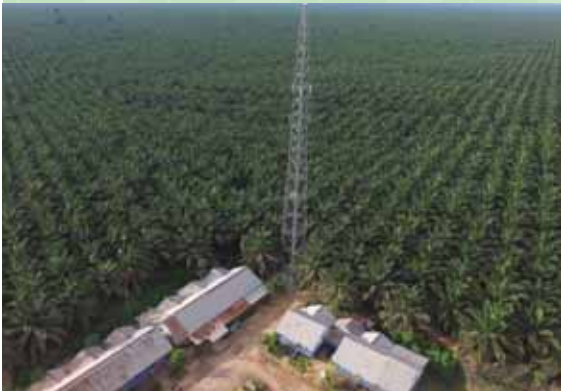
A telecommunication tower was erected through collaboration with local telecommunication company to provide communication access to our estate community
