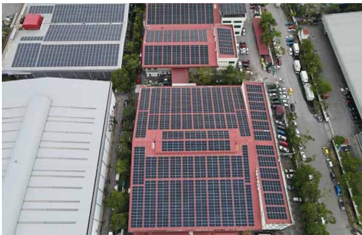
Solar panels installed on rooftops of the factory
