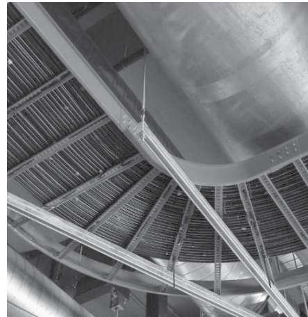
Electrical wiring system
