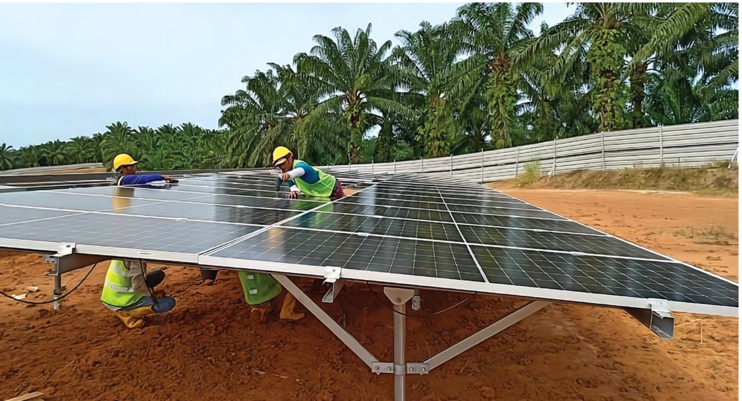
Vicinity view on installation of mock-up solar panel, 5.9MWa.c. Large Scale Solar Photovoltaic Plant in Tawau
