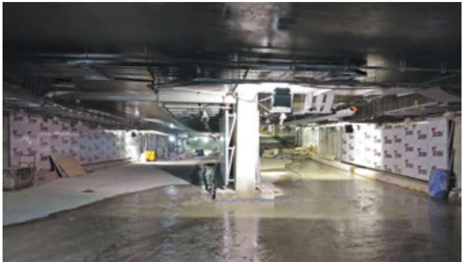
▲ TRX City Dispersal Road Tunnelling Link to Jalan Tun Razak, Kuala Lumpur
