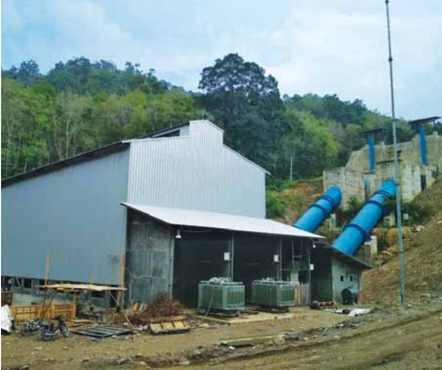
▲ Power House and Penstock at Lintau, Indonesia
