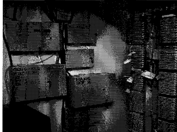
MDF room of a building where we performed inside plant installation and commissioning services
