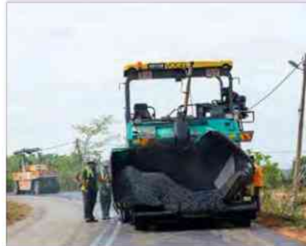
BDB Infra secured an RM204 million state road maintenance contract from the Kedah Government on 15 May 2023 based on its competence as a G7 Grade contractor. The contract was awarded based on BDB Infra's experience and an excellent track record in carrying out road maintenance and construction works in the northern part of the country.
