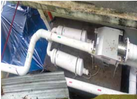
Photo 3: Rainwater Harvesting System - MAHA ESTET
