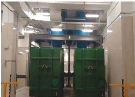
Photo 1: Automated Waste Collection System for Healthcare Waste Management Services
