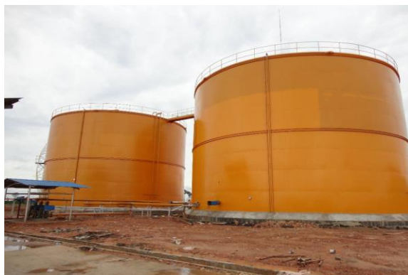
CPKO storage tanks
