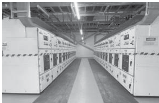
11kV medium voltage switchgear panel
