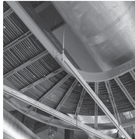
Electrical wiring system
