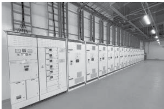
Low voltage main switchboard panel
