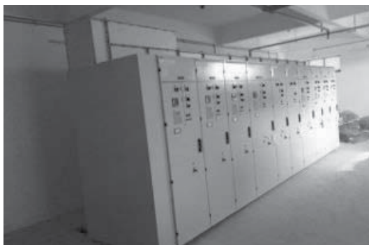
33kV medium voltage switchgear panel
