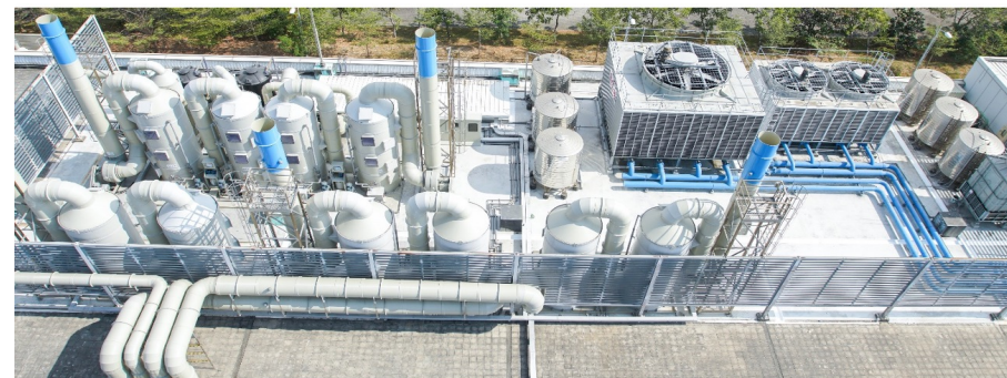
Continue to improve on the optimisation of energy conservation for our scrubbers, which are our single biggest user of electricity.
