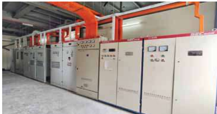
Picture: Control Room installed at Green Cement's grinding plant located in Kota Tinggi, Johor
