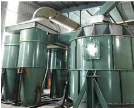
Picture: Cyclone and Classifier installed at Green Cement's Grinding plant located in Kota Tinggi, Johor
