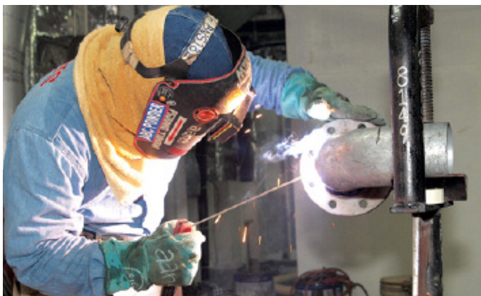
Another registered vendor, AANS Sdn. Bhd., doing piping work on board of PV3.
