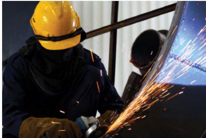
A skilled worker, cutting the steel for the construction of tug boat at Jerejak Yard.
